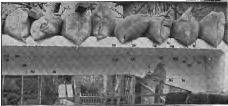
FIG. 186.—Beam I, Cracks and Rupture in the vicinity of the intermediate support.
