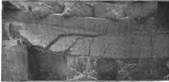
FIG. 134.—Beam I, cracks in the end without stirrups at the breaking load.
