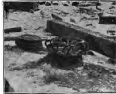
FIG. 270.—Station in Cannstatt. Head of pile which was driven without cap or driving block.
