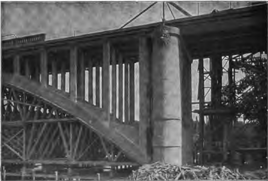
FIG. 300.—Highway bridge over the Isar near Grünwald. View of the left abutment.
