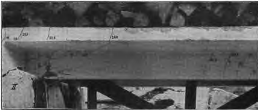
FIG. 187.—Beam II, Cracks and Rupture in the vicinity of the intermediate support.
