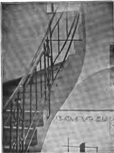
FIG. 240.—Winding reinforced concrete staircase without side strings in the Handel School in Landau.
