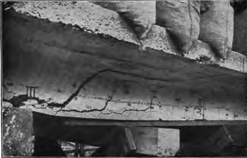
FIG. 136.—Beam III, with Thacher rods under the breaking load, at the end without stirrups.
