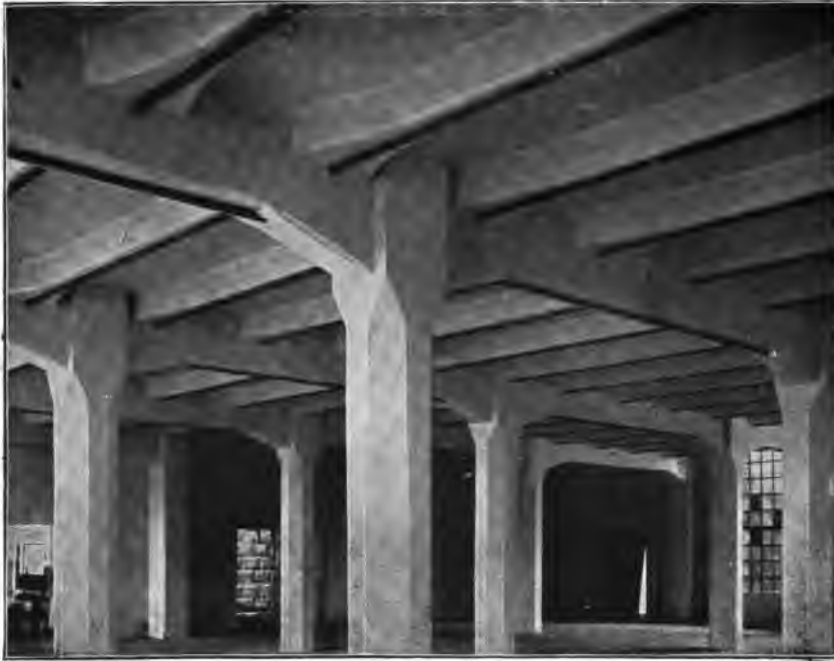
FIG. 229.—View of a floor in the Singer Manufacturing Co. factory showing widening of the beams where they intersect the girders. Columns of béton fretté.
