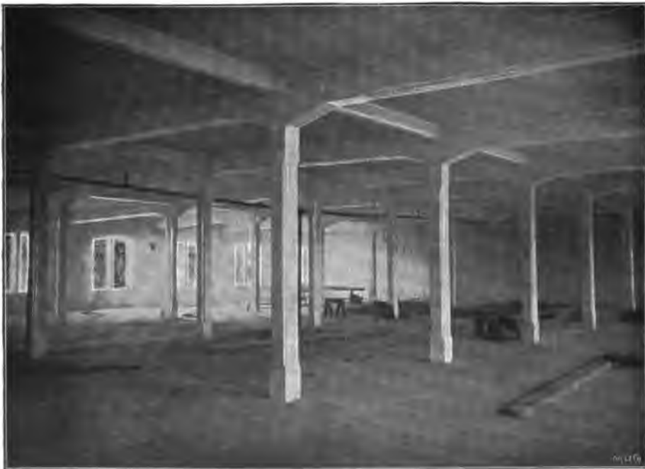
FIG. 207.—Spinning factory in Tammerfors (Finland), haunched floor slabs between girders, stiffening beams between the columns.
