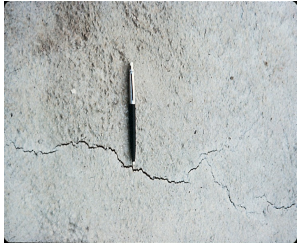
Figure 1: A typical plastic shrinkage crack. (Courtesy of Portland Cement Association)
